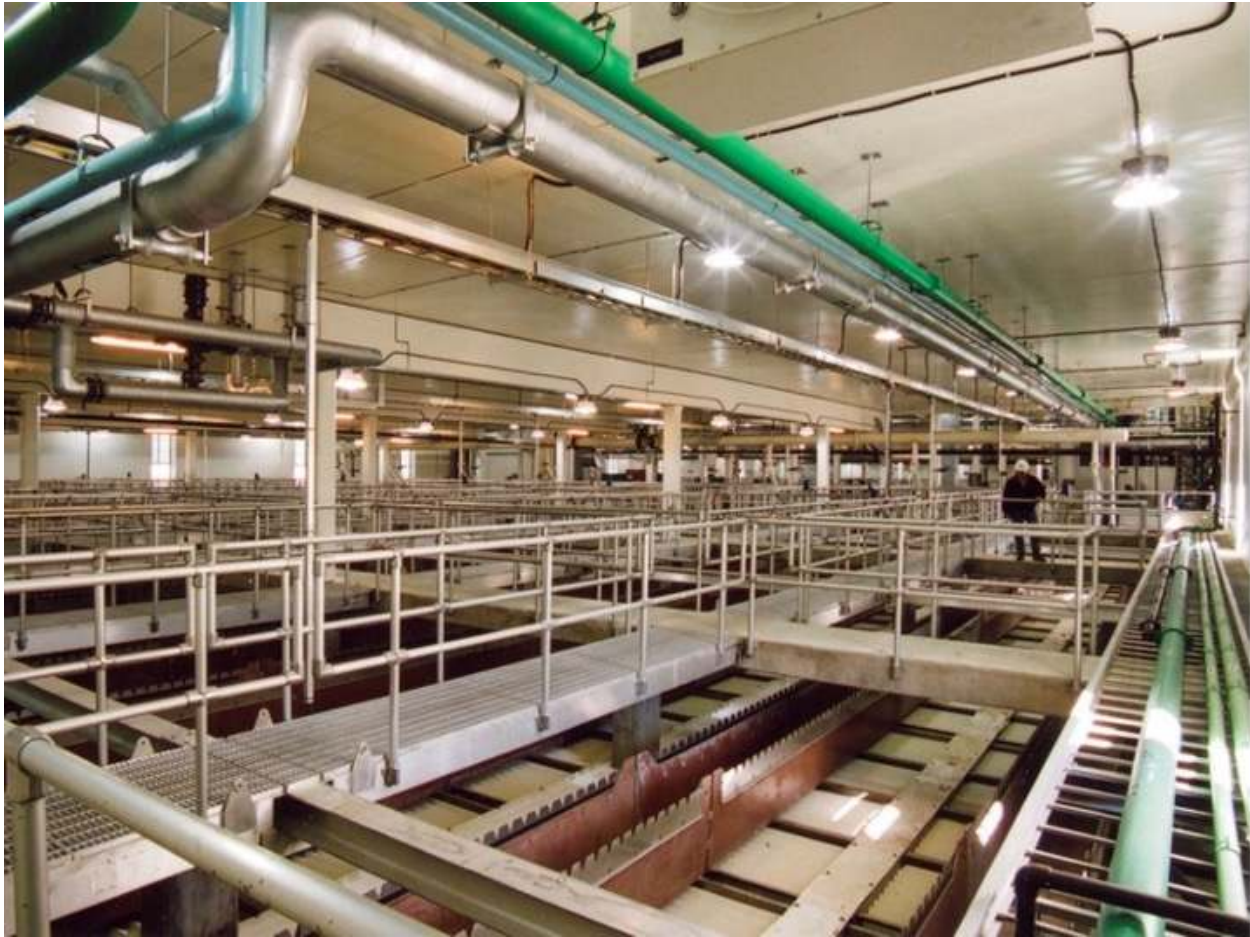
GOLD BAR WASTEWATER TREATMENT PLANT – ENHANCED PRIMARY TREATMENT TANKS
