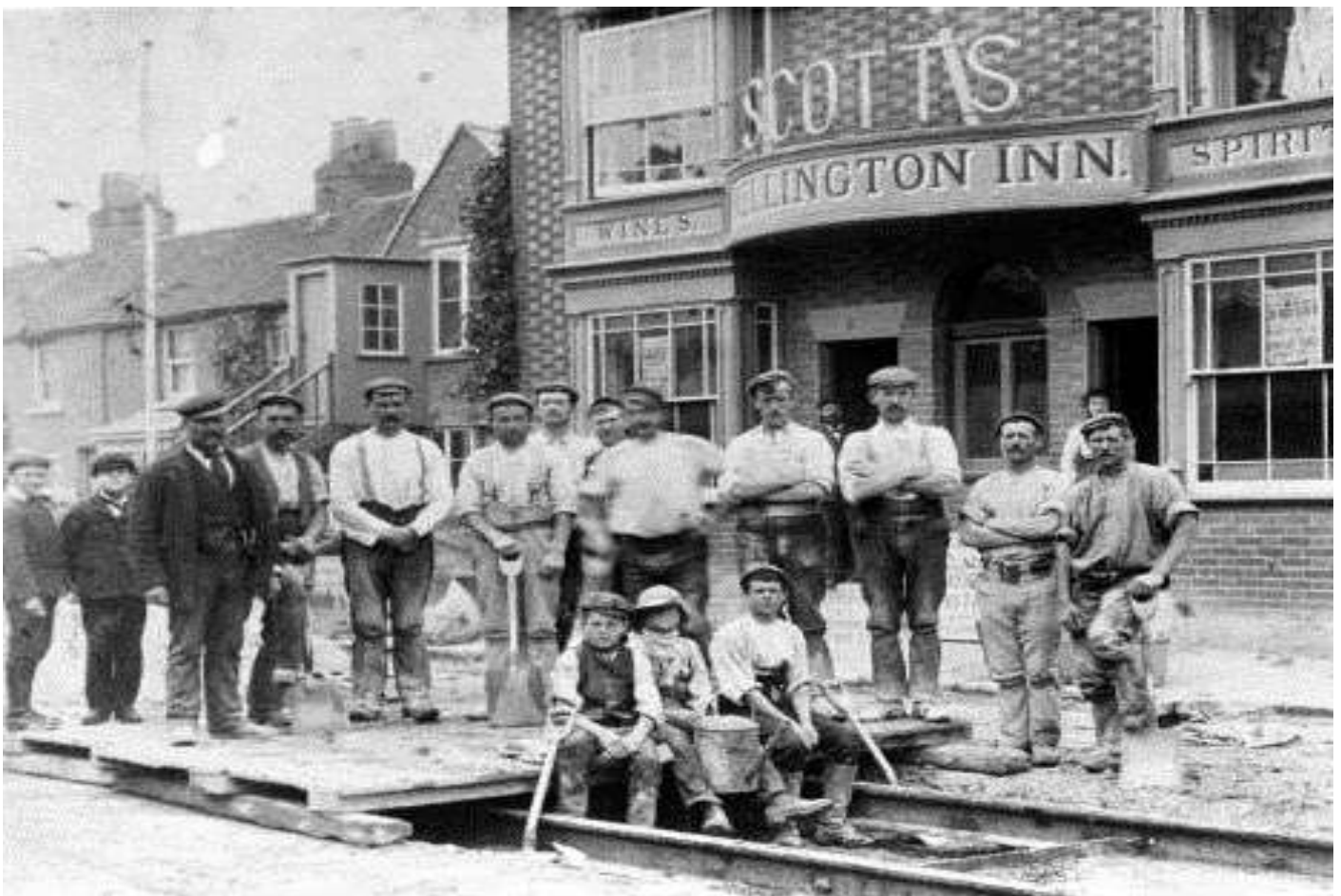
Workmen laying the track for the Portsdown and Horndean Light Railway, 1902. Richard Scott can be seen standing in the doorway of the Wellington Inn
